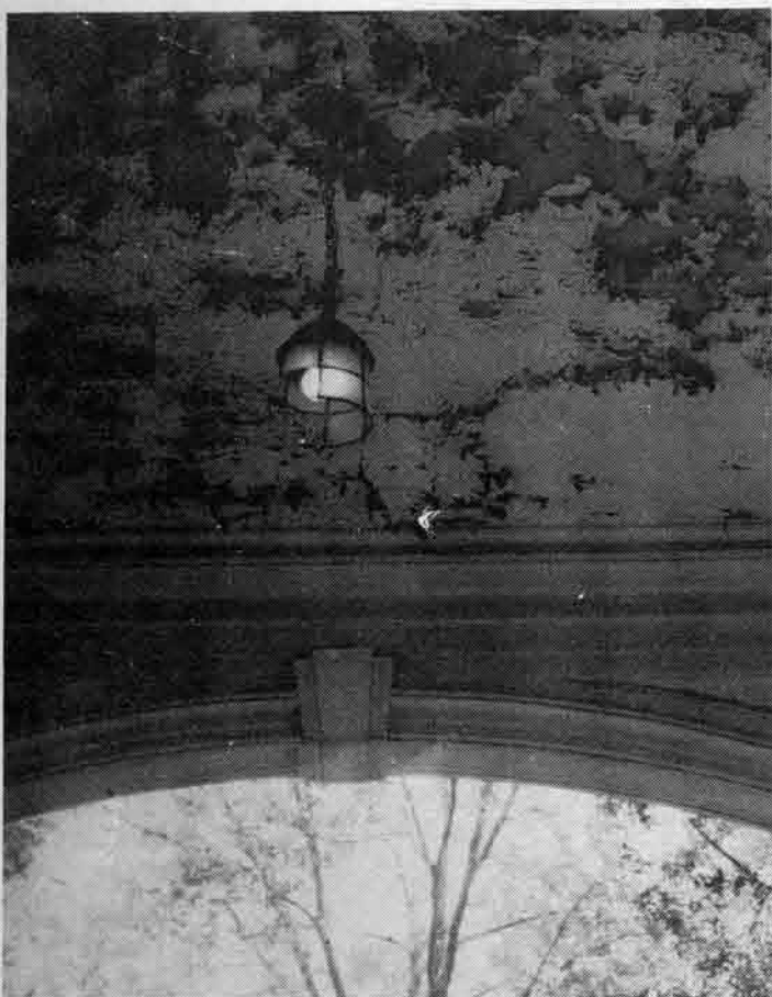
Paint peeling from porch of Administration bldg.
